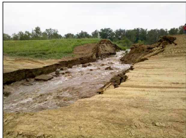
Levee failure in Hamburg, Iowa (Source: Iowa Department of Public Safety)
